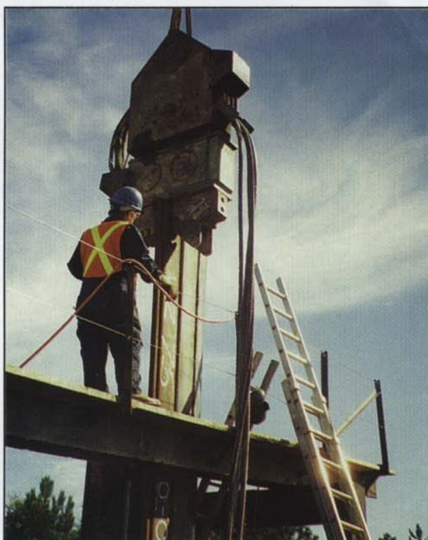
The Barrier was driven to refusal through stiff to hard soils comprised of a mixture of sand, clay and gravel using a crane-mounted vibratory hammer.
